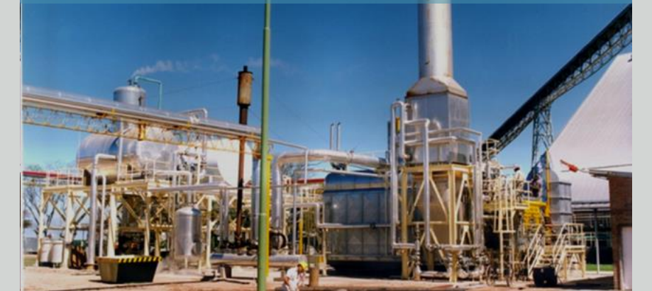
WATER INTAKE AND TREATMENT AND STEAM GENERATION LA PLATA CEREAL PUERTO SAN MARTIN, ARGENTINA
